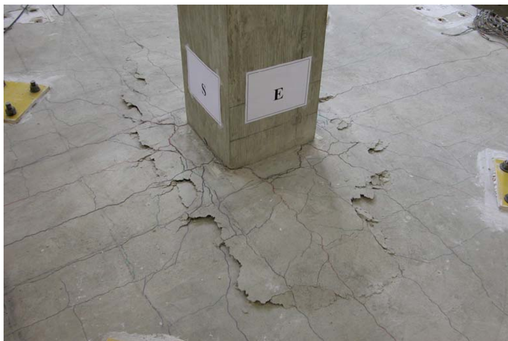
Figure B.1: Failure pattern of Specimen LG0.5.
